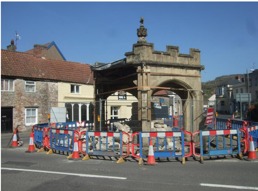
Fig 1: Cheddar market cross semi demolished by a private car for the second time in 12 years (2012)
