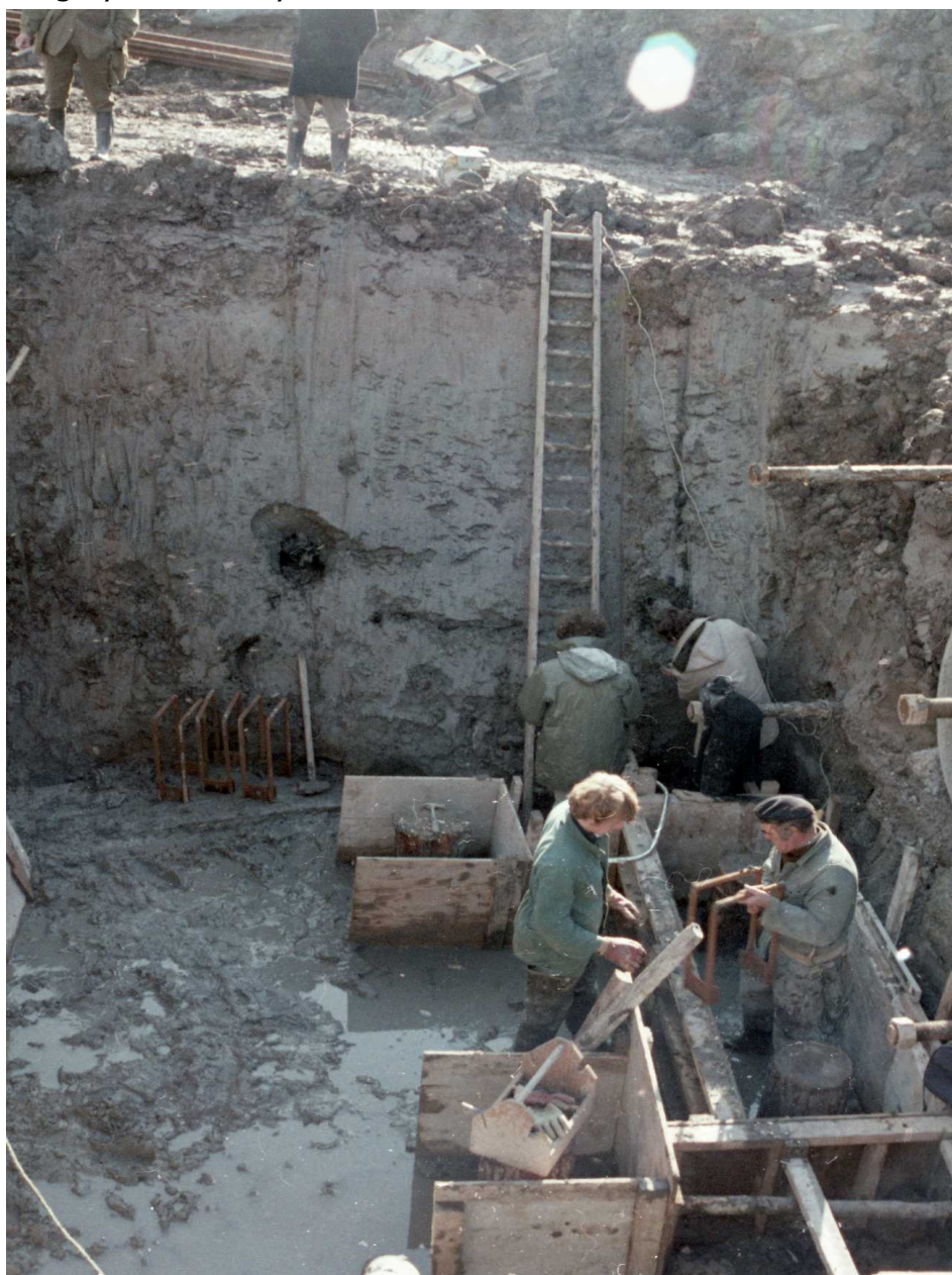
Fig 3: South face of the engineering excavation for the new sluice, 1982 Photo: Keith Gardner archive
