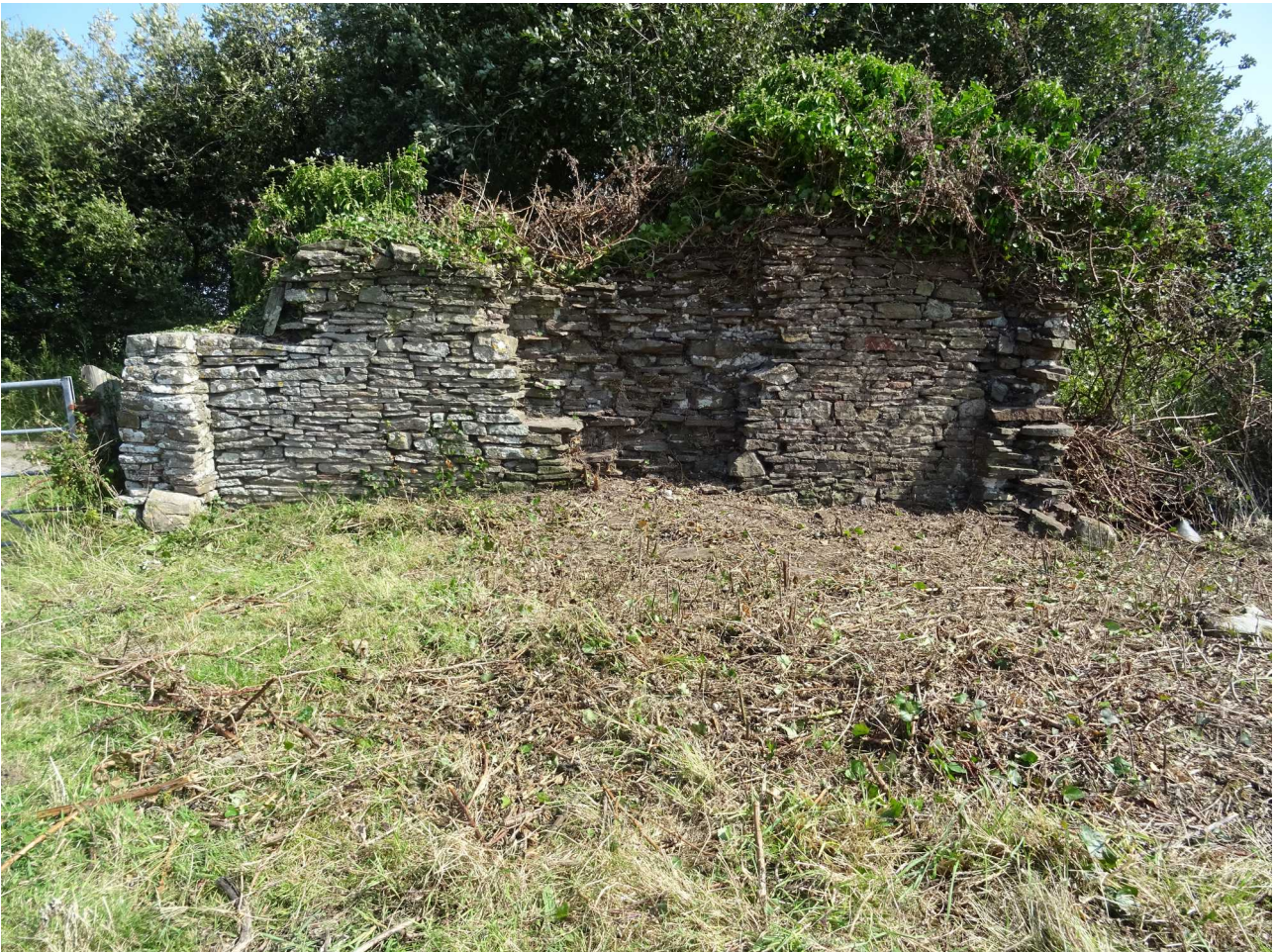
Surviving standing gable wall of Rose Cottage against the local lane
