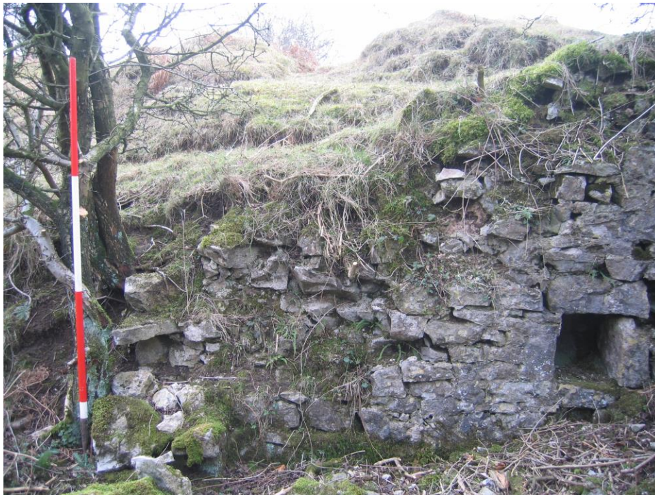
Fig 5: West cheek wall, from E, showing evidence of return at S end
