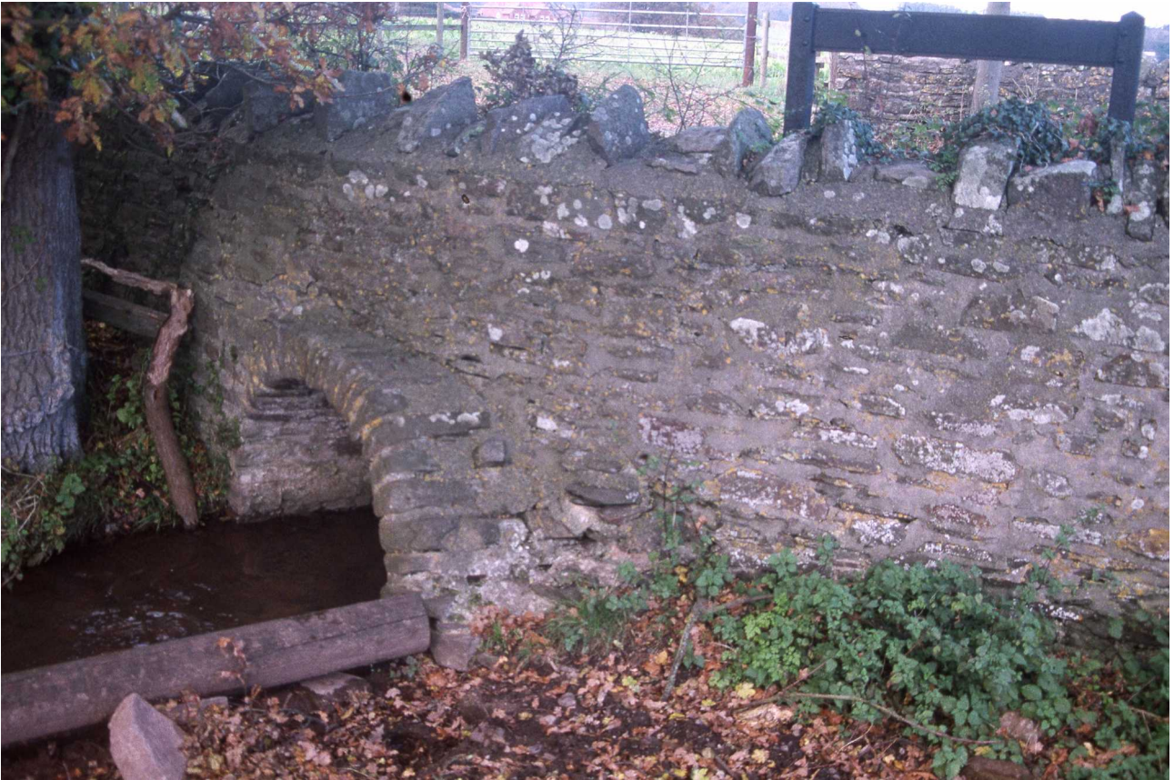
Fig 14: Backwell Bow, on the Backwell Common to Nailsea Road, over the upper Kenn River. Note the curious mismatch between 'tunnel' and parapet, presumably due to cack-handed rebuilding
