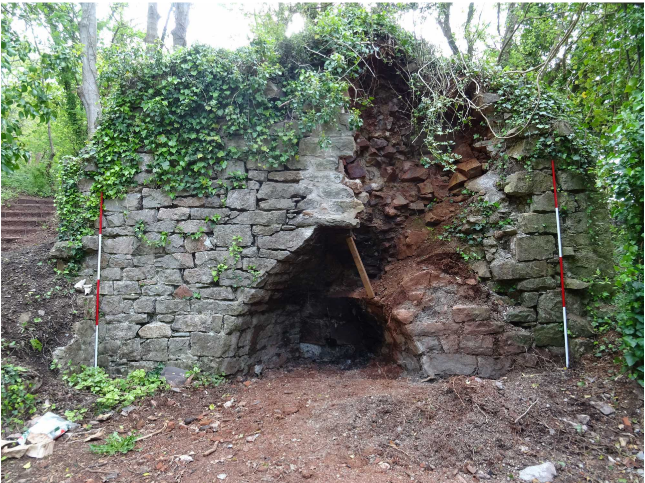
Front elevation of the western limekiln at Prestow Wood before conservation repair
